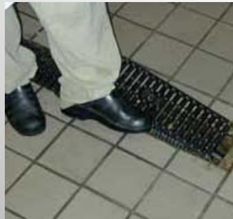
Replace drain covers and keep drains clear of debris.
