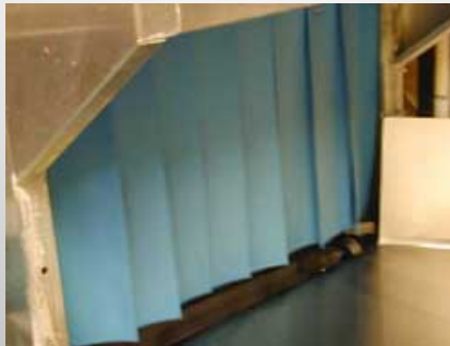
Dishwasher guarded to prevent accidental scalding
