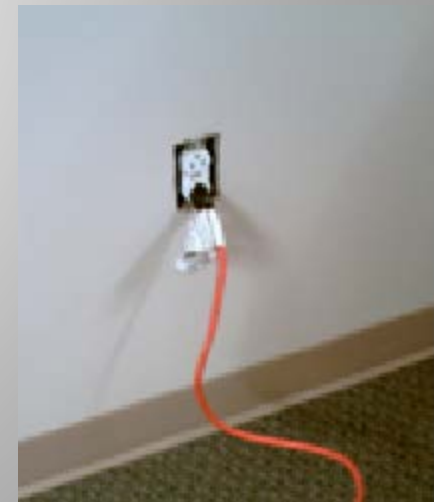
Missing Plug Plate
