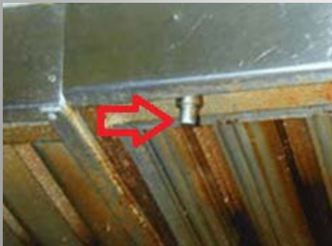
Gas extinguishing System over hood
